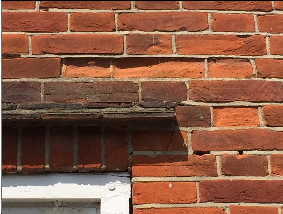
Example of damage caused due to cement pointing.
